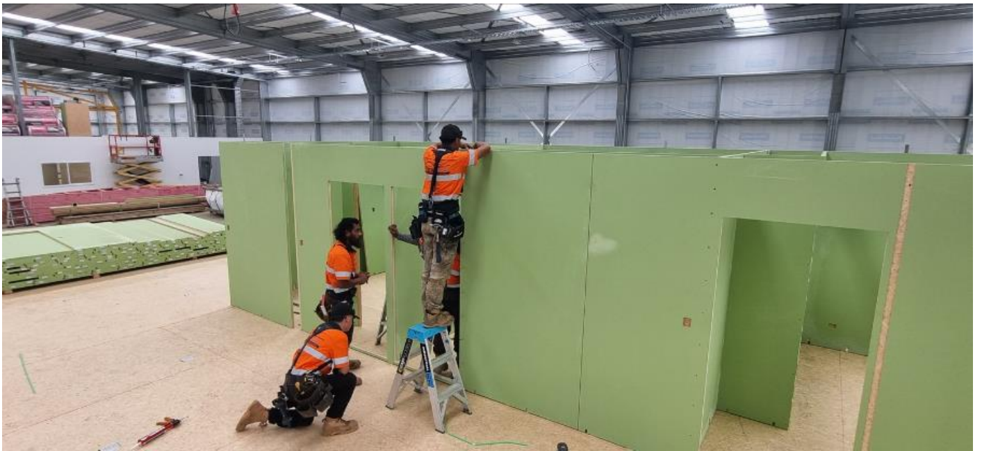
Above the team ensures the Panels are squared off at the top.
